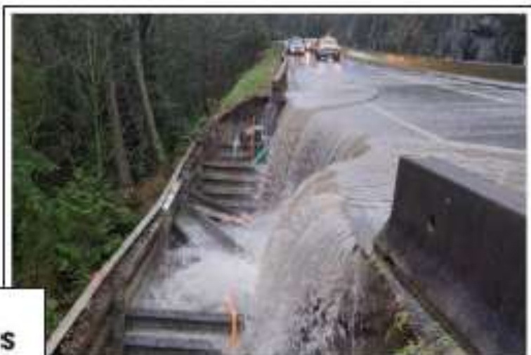
During the 2021 atmospheric river event, the United portion of the Trans-Canada Highway (File courtesy: Enrico Serrano Inc.)
